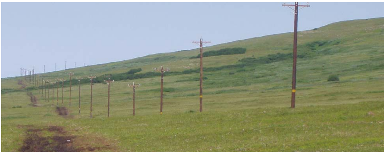
Toksook Bay to Nightmute 13.8 kV intertie. Photo courtesy of Denali Commission.
