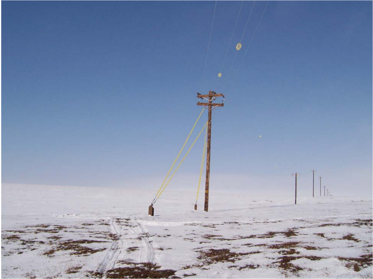
Toksook Bay to Nightmute 13.8kV intertie. Photo courtesy of Alaska Village Electric Cooperative.
